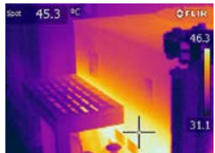
Fig. 7—Low operating fluid level in reservoir
